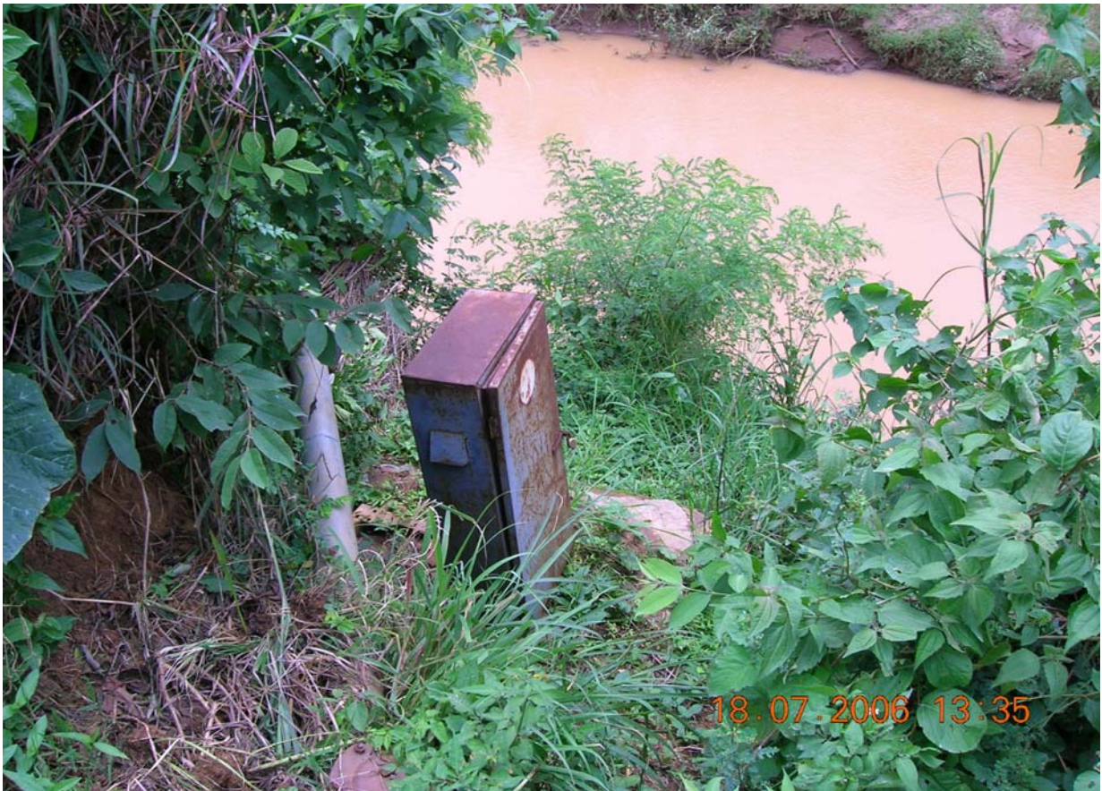
Photograph – 1: BKVY Lift Point of OLIC at Malimurla, Similiguda, Koraput
