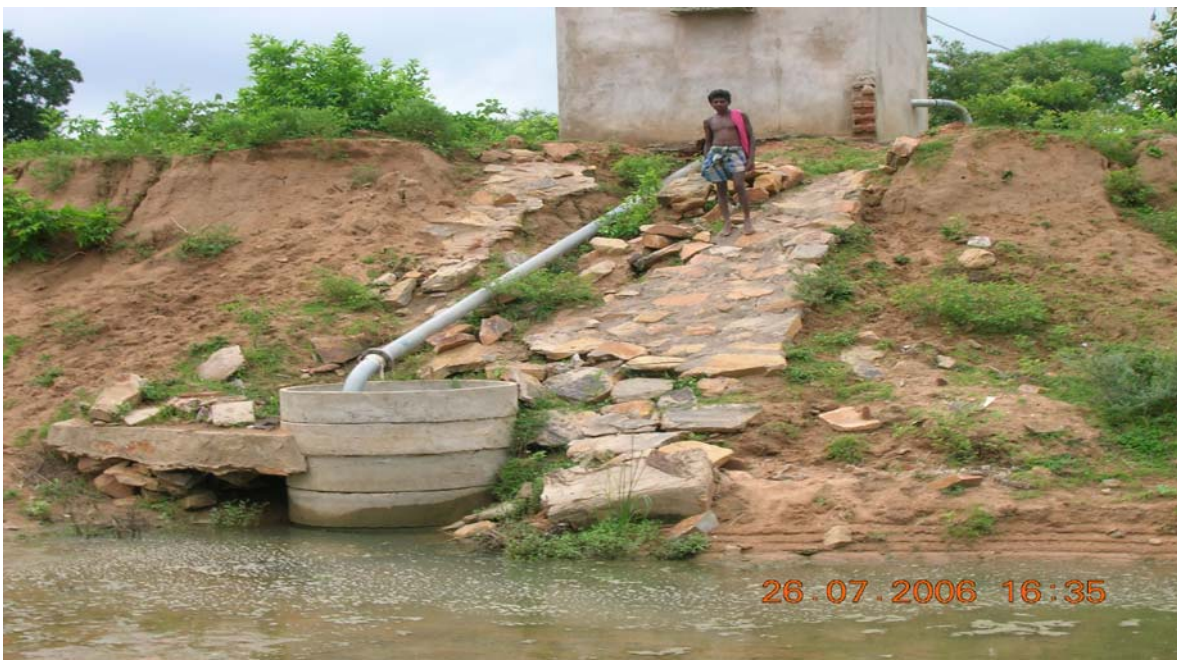
Photograph – 2: BKVY Lift Point of OAIC at Krishna, Komana, Nuapada
