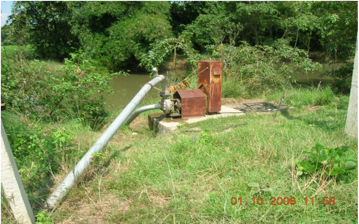
Photograph – 5: BKVY Lift Point of OLIC in Binka, Sonapur
