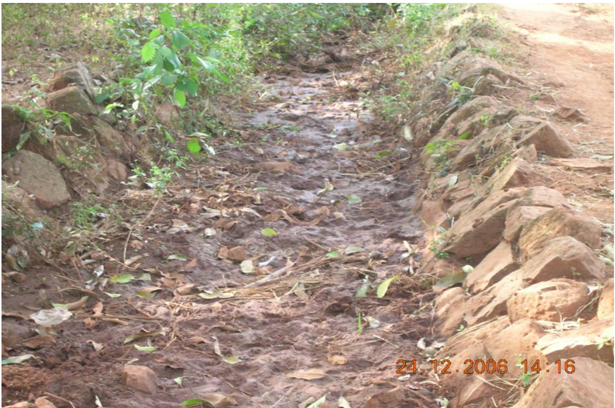
Photograph – 12: A Poorly maintained minor canal of BKVY MI project in Nandpur, Koraput
