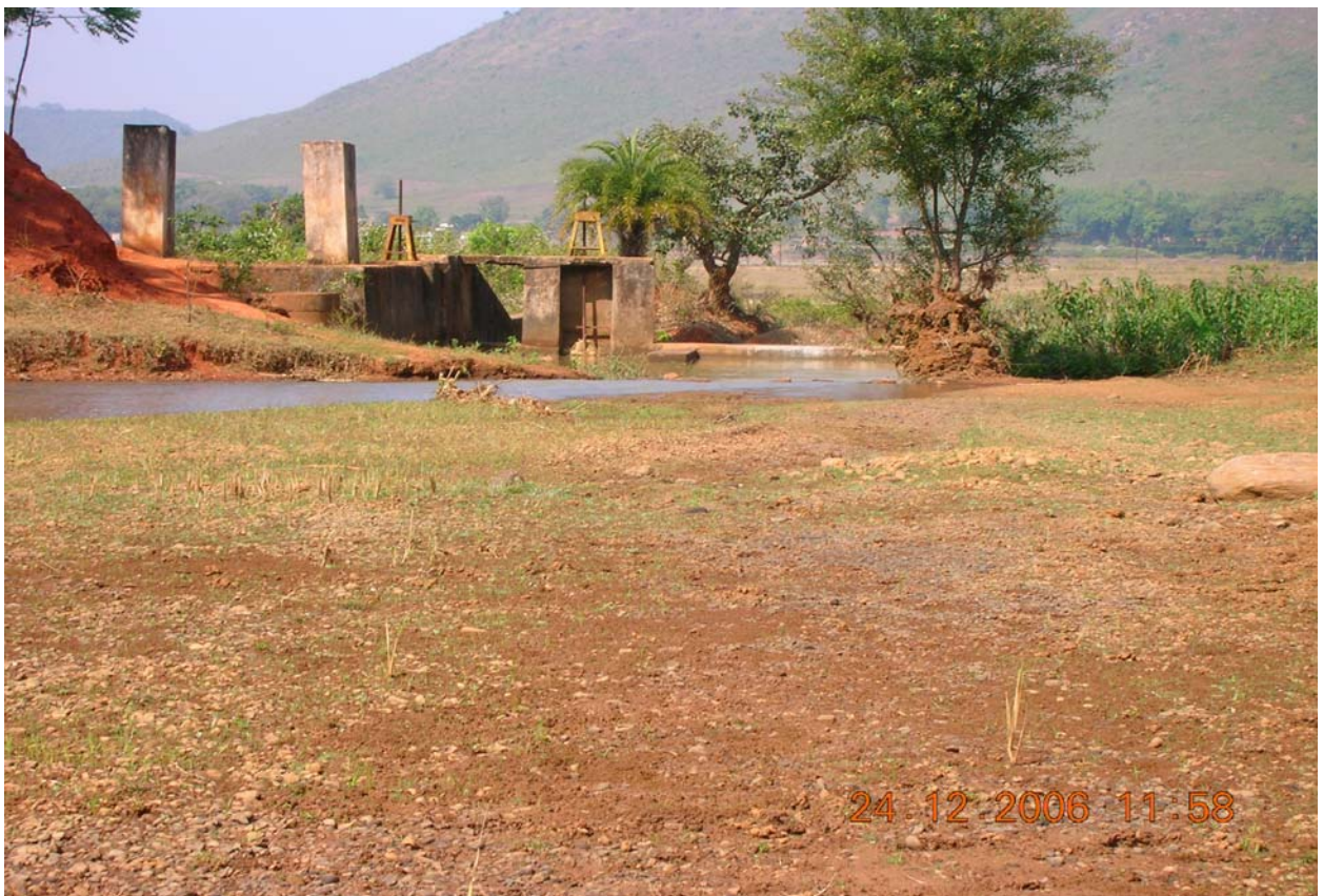
Photograph – 8: Poorly maintained BKVY MI Project at Nandpur, Koraput
